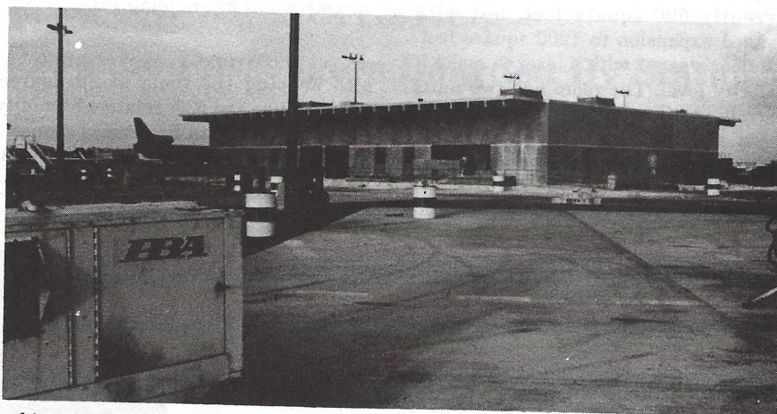
Looking at the new Miami terminal from the west ramp side, it is evident that the building is nearing completion.
